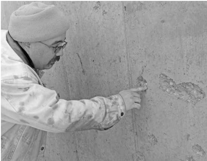
2018.01.06 Damage to Multi Purpose Bay 1 Damage to concrete wall by shooter not taking account where their bullets are going after hitting the target.
